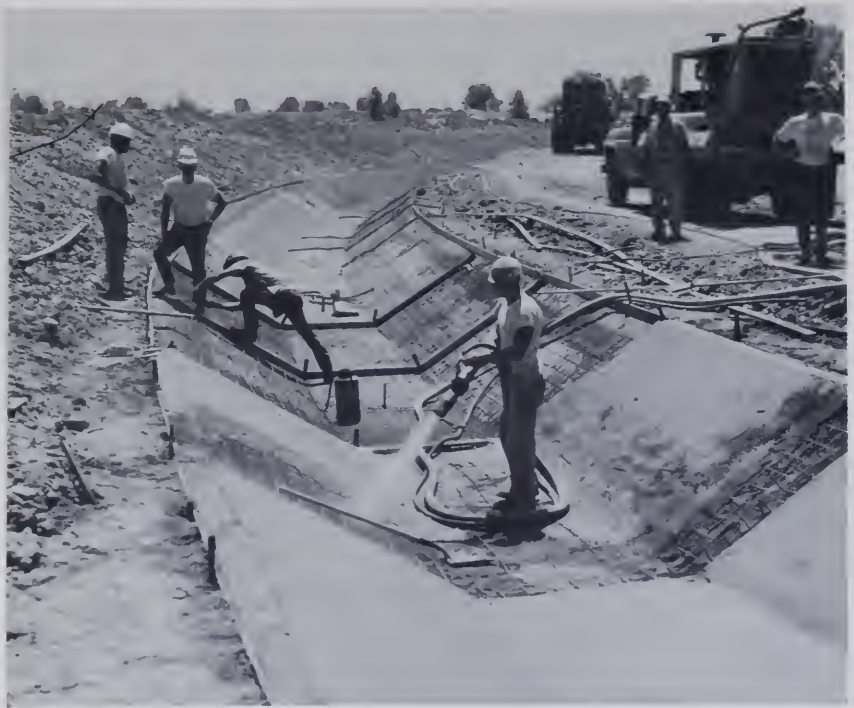
Figure 204.—Shotcrete being applied to canal prism with wire mesh reinforcement installed in the Auburn-Folsom South Canal, Central Valley Project, California. P859-245-5383.
